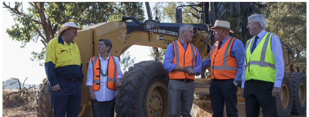
ON THE ROAD: Inspecting the work on the widening The Bogan Way with (from left) Cr Barbara Newton is Jason Bliss, Civil Construction team, Parkes Shire Council, Parkes Deputy Mayor Barbara Newton, recently retired New South Wales Parliamentary Secretary for Natural Resources and Western NSW Rick Colless MLC and Steven Campbell, Director of Planning, Parkes Shire Council.
