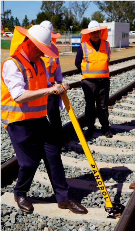
MOMENTOUS: Putting the final pin in place at Peak Hill to mark the completion of the Parkes to Narromine section of the Inland Rail. INSET: The gold commemorative pin.
