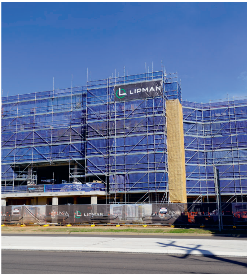
UNDER CONSTRUCTION: The UNSW Biomedical Sciences Centre in April 2024, having reached the highest point of its construction. Construction of the project was undertaken by Australian-owned family business Lipman.
